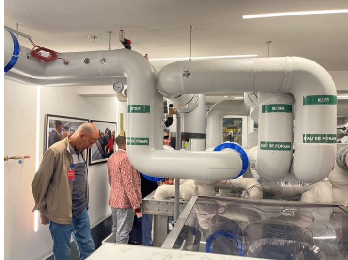
Figure 1- Visit of a shallow geothermal surface installation. “Eau de forage”: water from well, “eau froide primaire”: primary cold water, “aller”: forward, “retour”: return.
